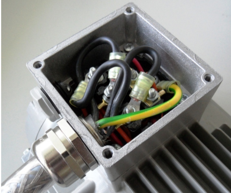
Fig. 22: Wiring on the motor connection box
